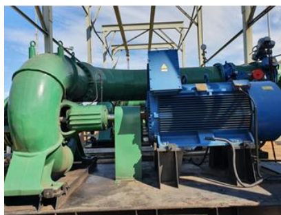
Gambar 3.1 Pompa Main Sea Water Pump (Sumber : PT Krakatau Daya Listrik,2020)
